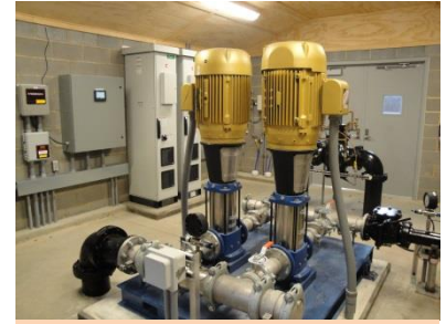
Inside the new Sycamore Rd. Booster Pump Station
