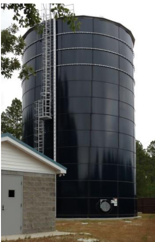
New Sycamore Road Booster Pump Station
